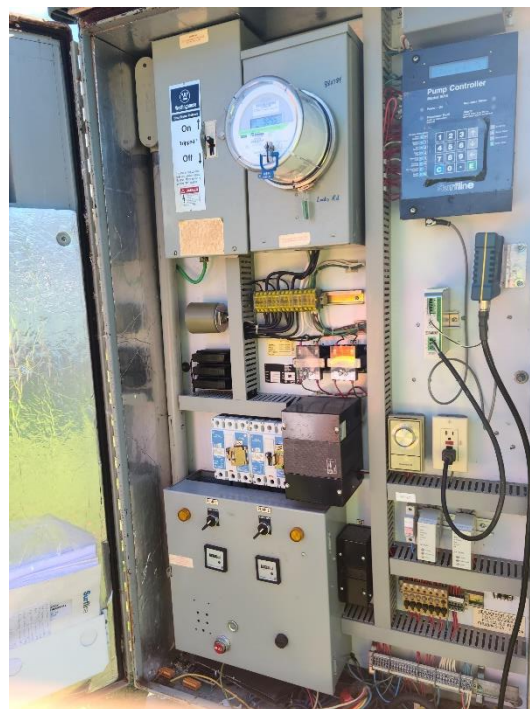
LS #5: Locks Road - Control Panel
