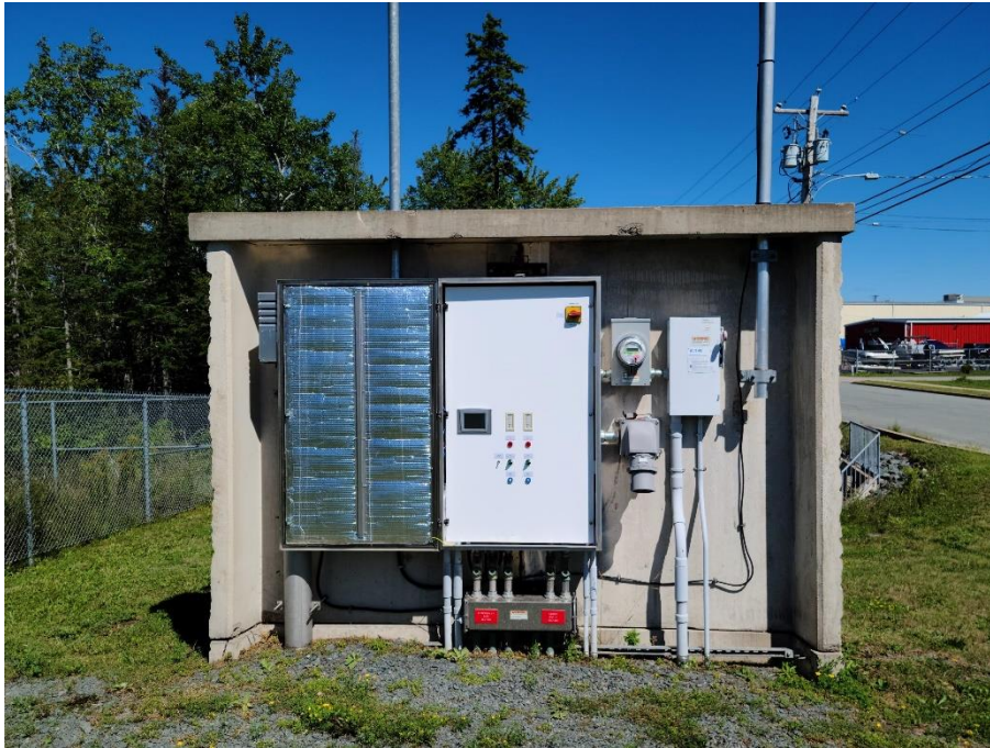
LS #11C: Park Road Extension - Pedestal & Control Panel
