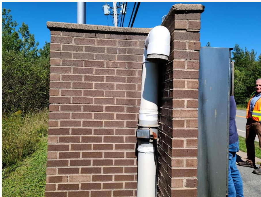
LS #14: Sportsplex - Pedestal with detached ventilation pipe
