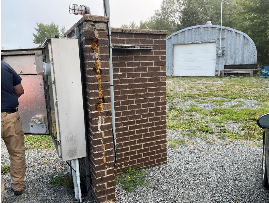
LS #17: Old Public Works Shed - Pedestal damage
