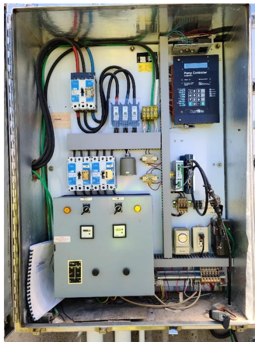
LS #11A: Industrial Park - Control Panel
