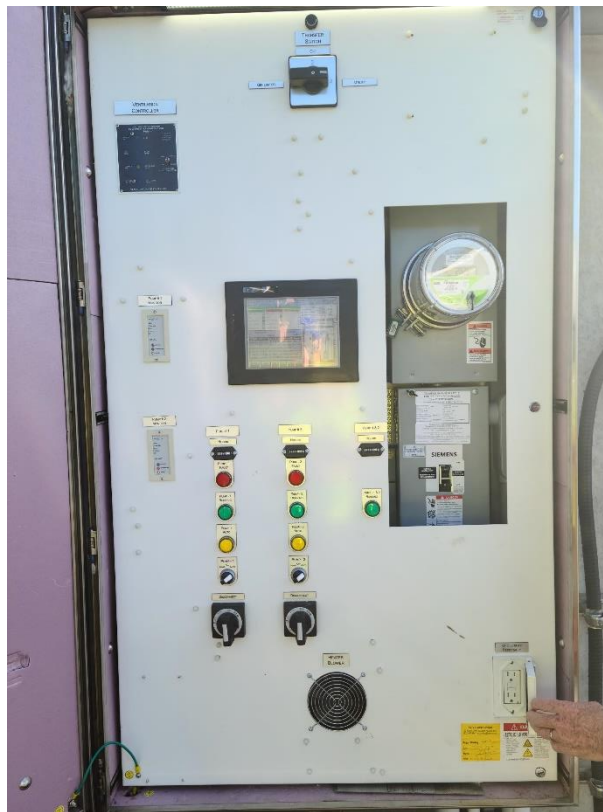
LS #2: Sherwood Park - Control Panel
