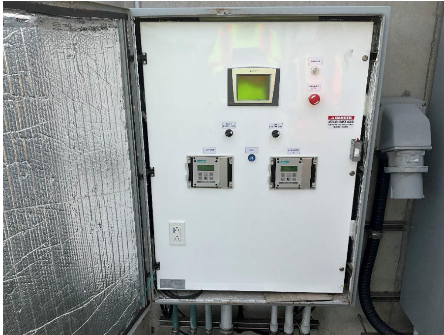
LS #24: Burgess Road - Control Panel
