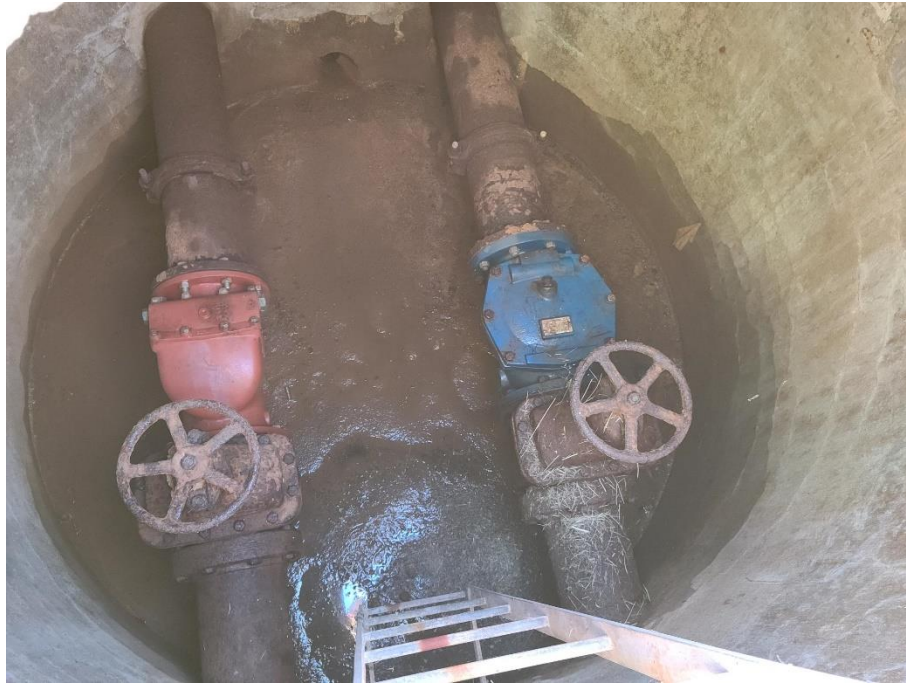
LS #14: Sportsplex - Inside of Valve Chamber
