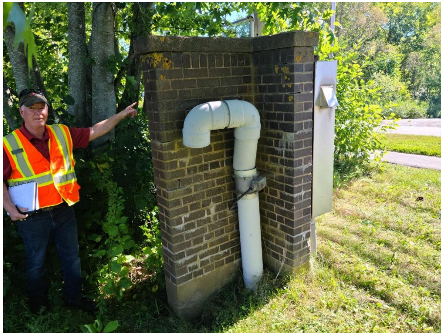
LS #9: Firehall - Pedestal in need of repair
