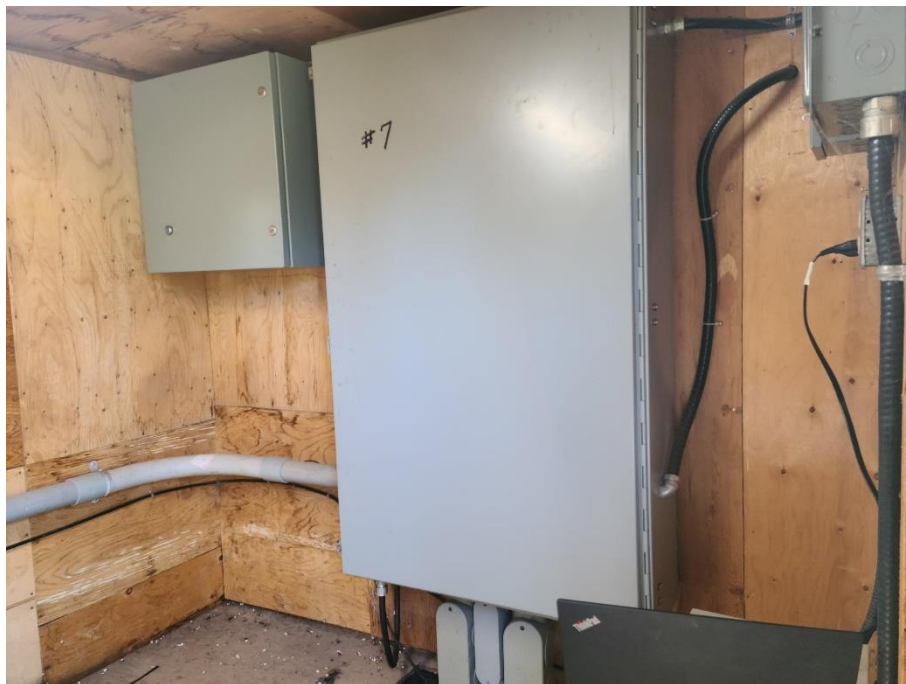
LS #7: Curley Portables - Control Panel inside of building
