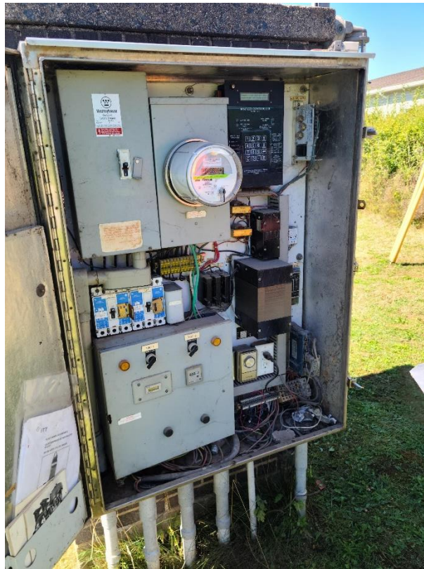
LS #10: Medical Centre - Control Panel
