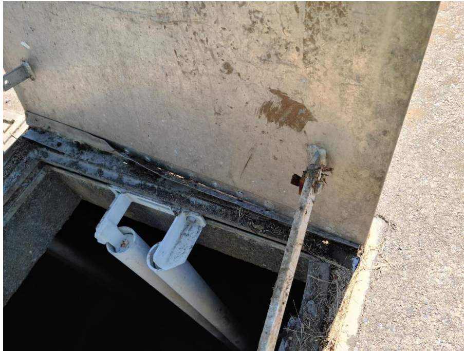
LS #11A: Industrial Park - Broken Hinge
