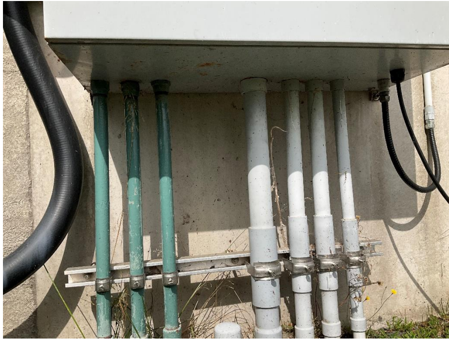
LS #23: Maitland Road: Conduit entering control panel
