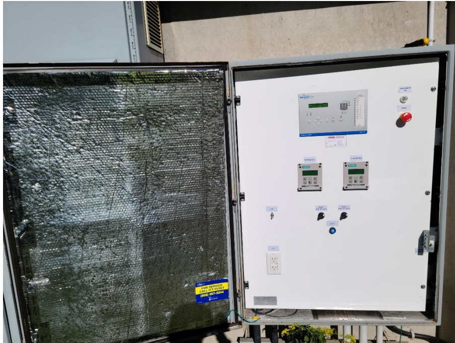
LS #4: Donaldson Ave - Control Panel
