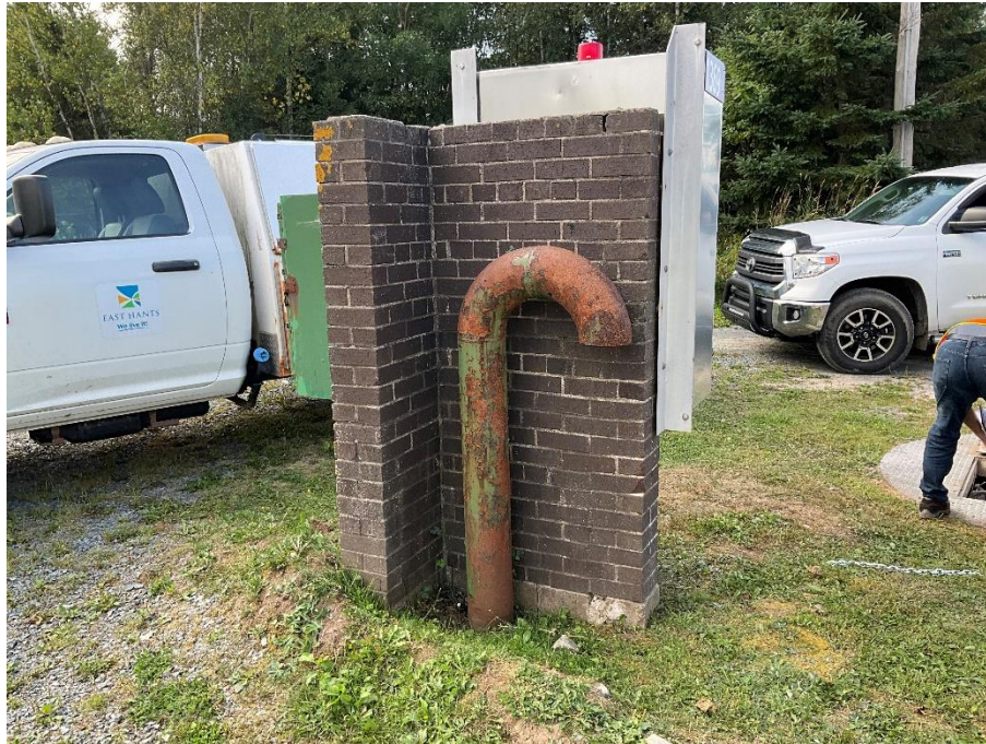
LS #18: Barney Brook - Pedestal with rusty ventiation pipe
