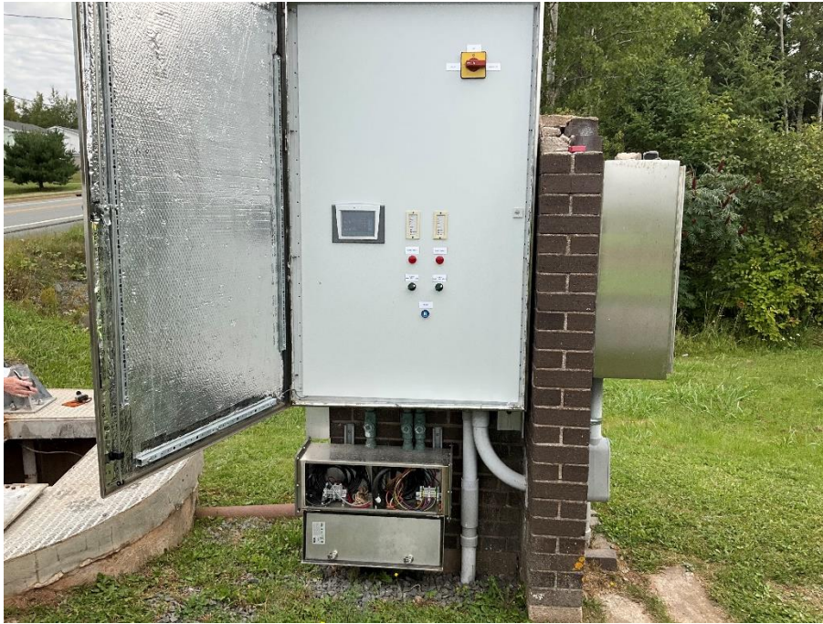
LS #20: Ross' Hill - Control Panel and unlockable electrical box
