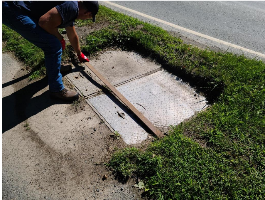
LS #9: Firehall - Damaged hatch cover
