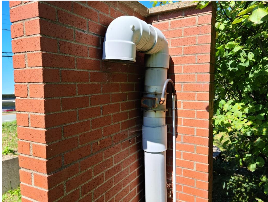
LS #12: Elmsdale Legion – Pedestal & detached ventilation pipe
