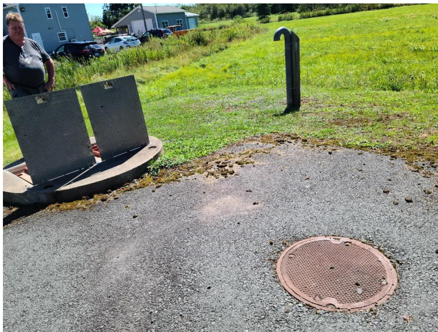
LS #11B: Carmies Daycare - Valve chamber and wet-well
