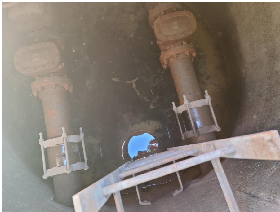
LS #8: Mill - Inside of Valve Chamber
