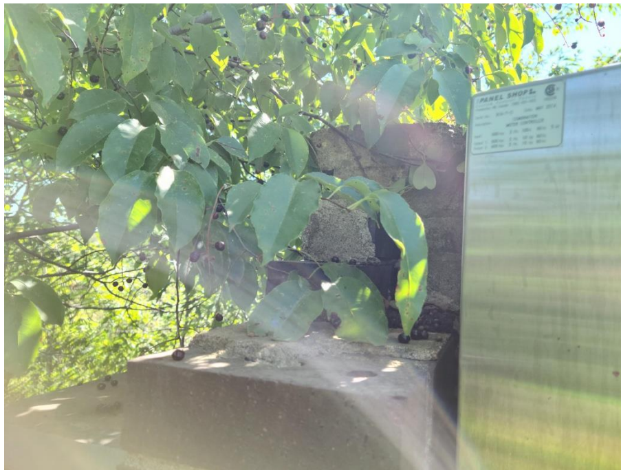
LS #16: Paley Road - Pedestal damage
