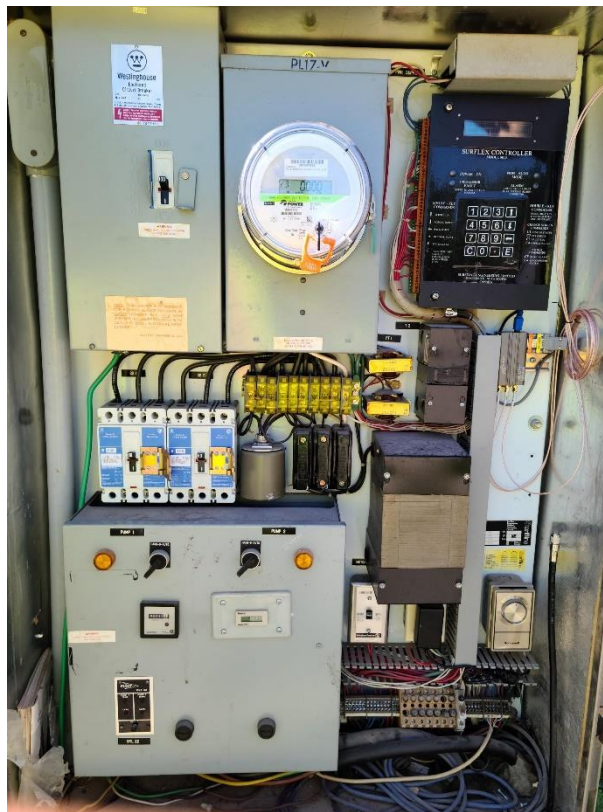
LS #14: Sportsplex: Control Panel
