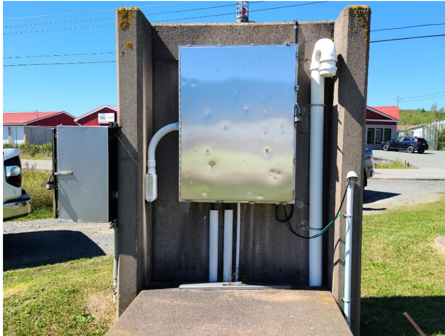
LS #11A: Industrial Park - Pedestal and Control Panel Enclosure
