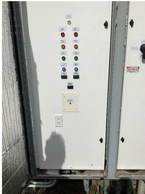
LS #23: Maitland Road - Control panel
