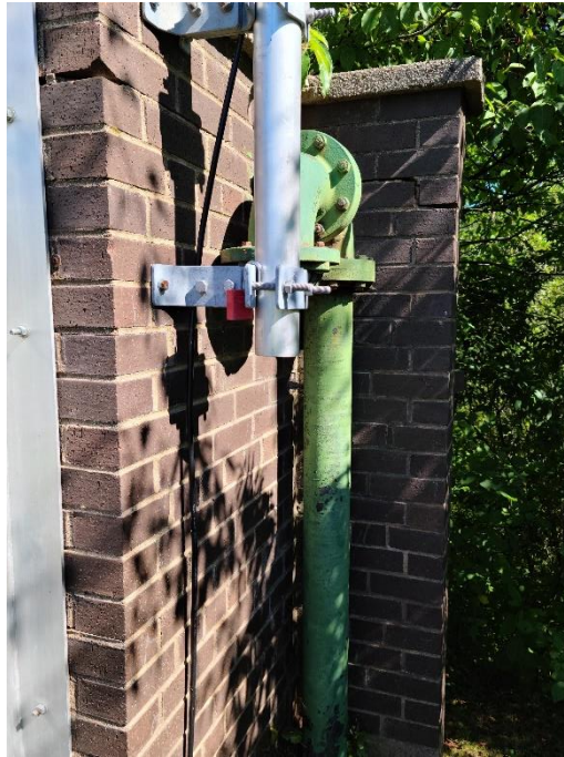
LS #16: Paley Road - SCADA mast attached to brick pedestal
