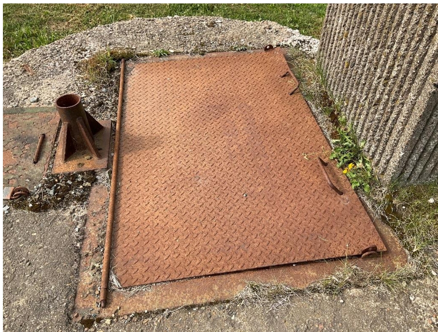
LS #21: Main Office - Rusted hatch cover
