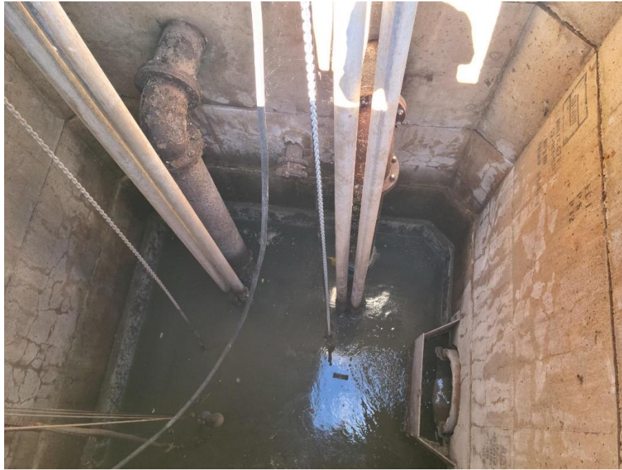
LS #14: Sportsplex - Inside of Wet-Well
