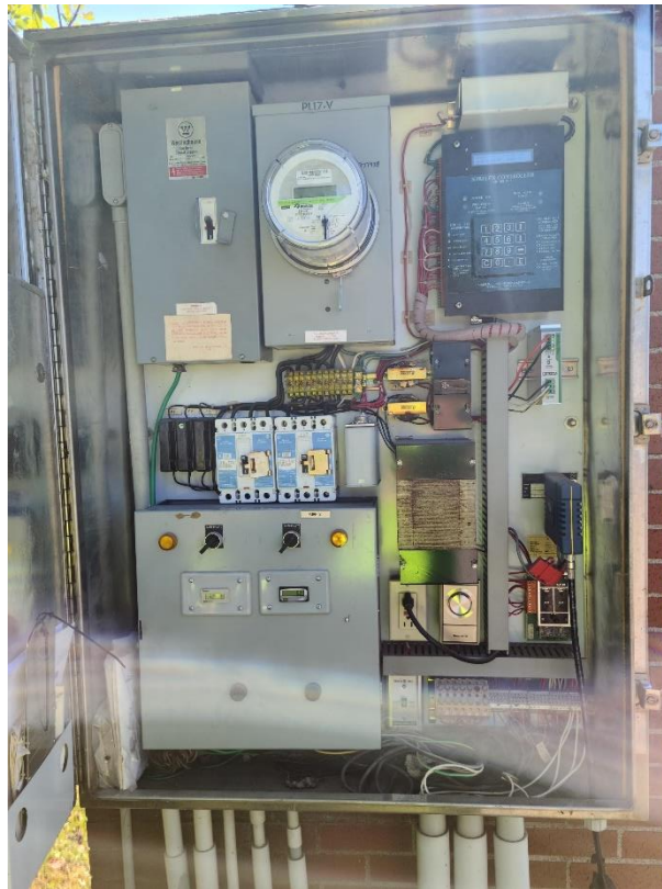
LS #12: Elmsdale Legion - Control Panel
