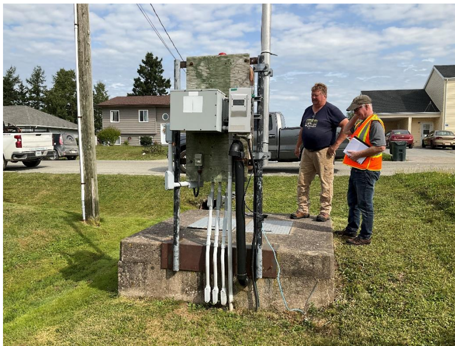
LS #22: Havenwood Road - Conduit from wet-well to control panel
