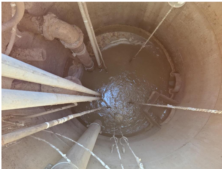
LS #4: Donaldson Ave - Inside of Wet-Well
