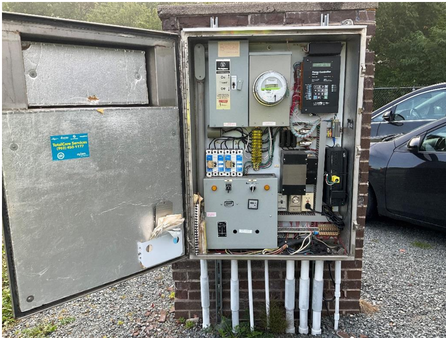
LS #17: Old Public Works Shed - Control Panel
