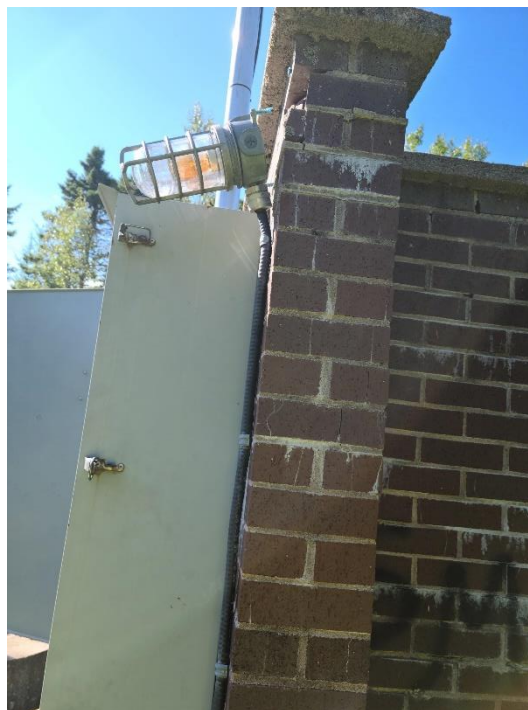
LS #15: Poplar Drive - Pedestal with hanging alarm light
