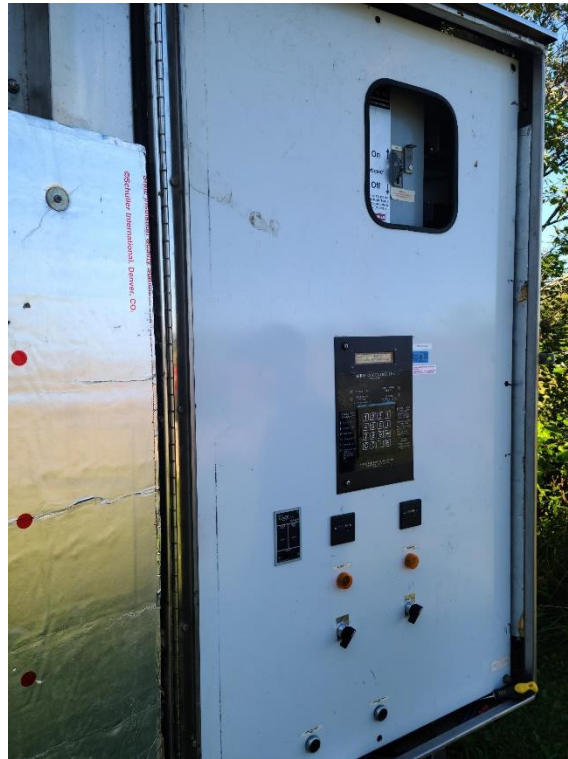
LS #3: Horne Settlement - Control Panel
