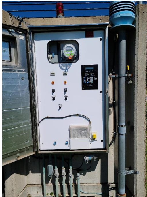
LS #11B: Carmies Daycare - Control Panel & Pedestal
