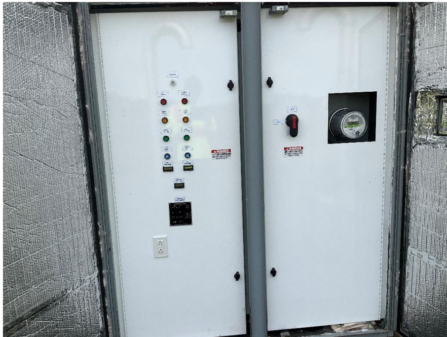
LS #24: Burgess Road – Monitor Panel and Power Meter
