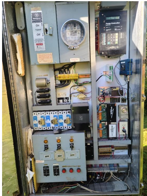
LS #1: Peter Horne Station - Inside of Control Panel
