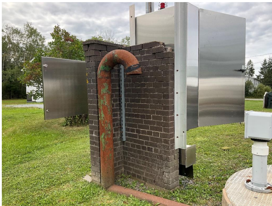
LS #20: Ross' Hill - Damaged pedestal and rusty ventilation pipe
