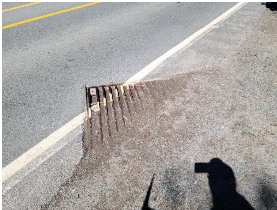
LS #11: Old Elmsdale School - Wet-Well hatch cover in roadway
