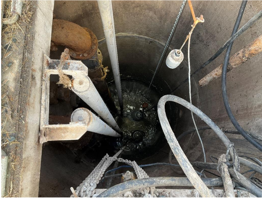
LS #18: Barney Brook - Inside of Wet-Well
