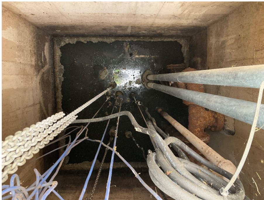
LS #22: Havenwood Road - Inside of Wet-Well
