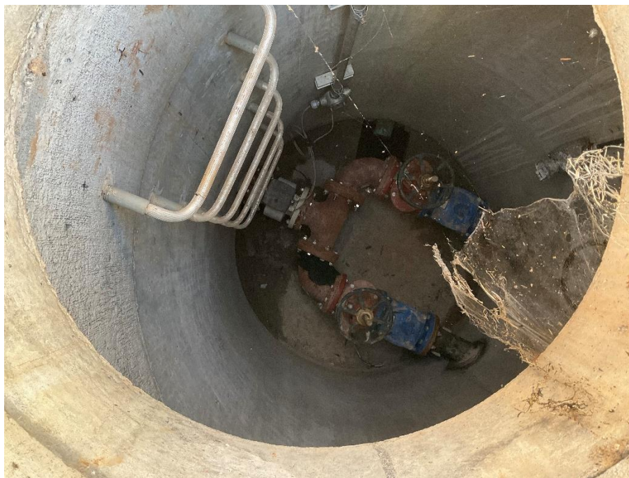
LS #19: Isenor Road - Inside of Valve Chamber
