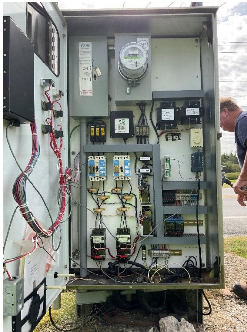
LS #21: Main Office - Control Panel
