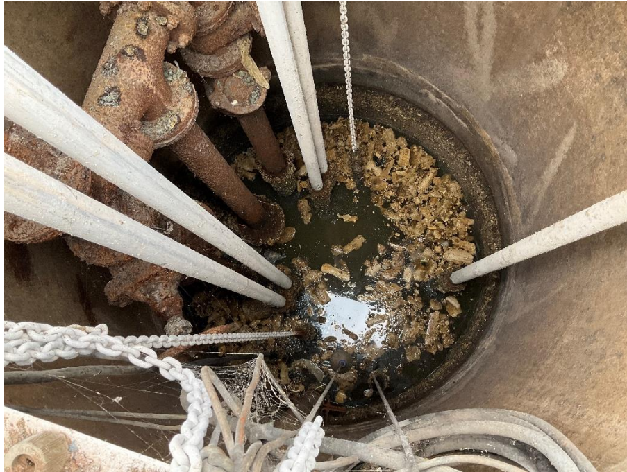
LS #20: Ross' Hill - Inside of Wet-Well
