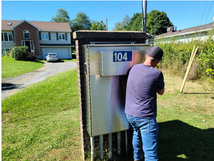
LS #10: Medical Centre - Pedestal and Control Panel Enclosure
