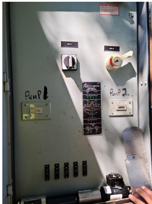
LS #10A: Pine Grove: Control Panel
