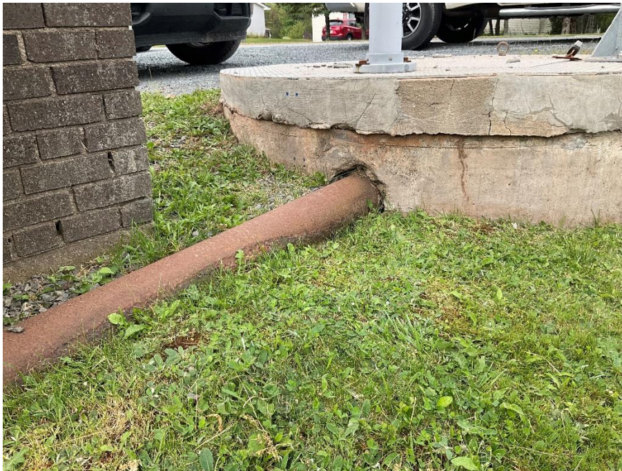
LS #20: Ross' Hill - Concrete eroded from around ventilation pipe
