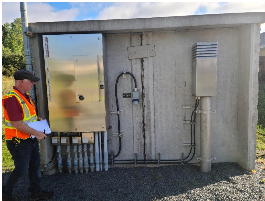
LS #2: Sherwood Park - Control Panel & Pedestal
