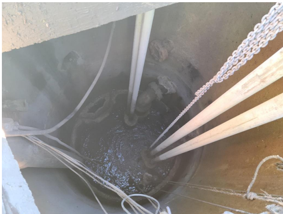
LS #9: Firehall - Inside of Wet-Well
