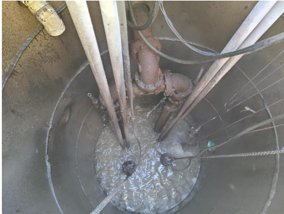
LS #11A: Industrial Park - Inside of wet-well. Note blowout from leaking check valve
