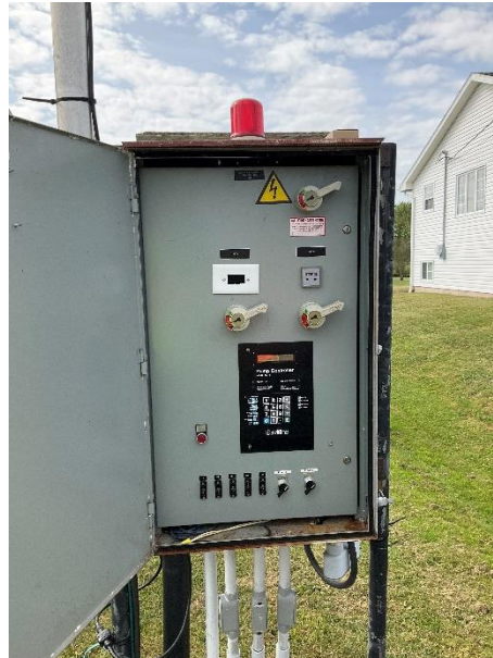
LS #22: Havenwood Road - Control Panel
