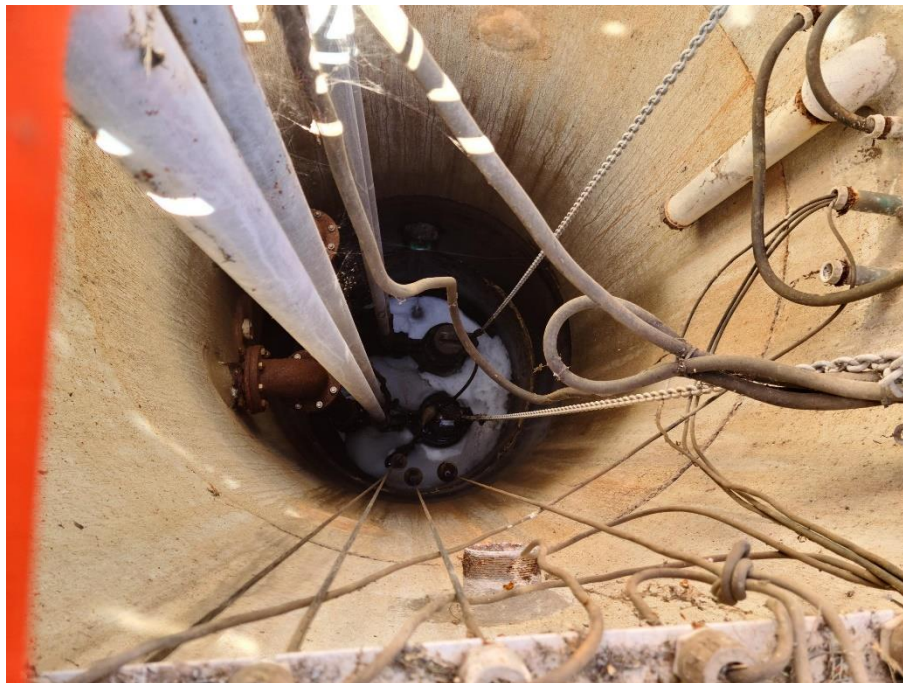
LS #11B: Carmies Daycare - Inside of Wet-Well
