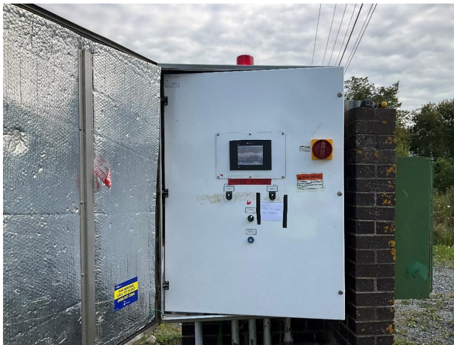
LS #18: Barney Brook - Control Panel
