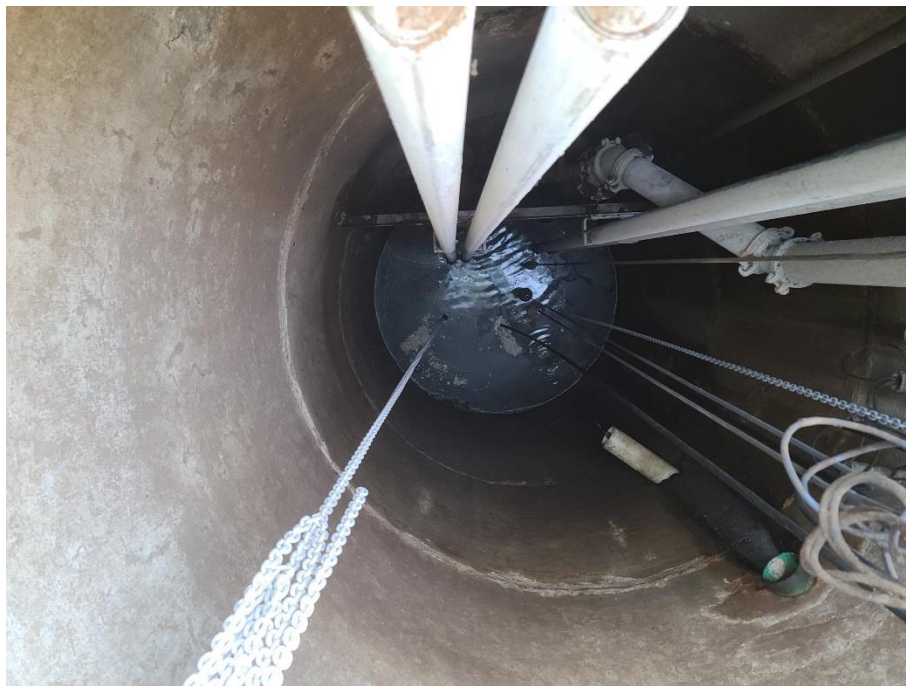
LS #1: Peter Horne Station - Inside of Wet-Well
