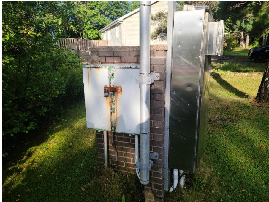
LS #1: Peter Horne Station: Pedestal & Control Panel
