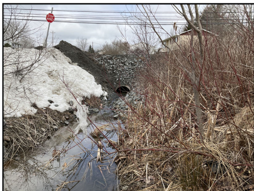
Photo 1: Flow out of outlet
