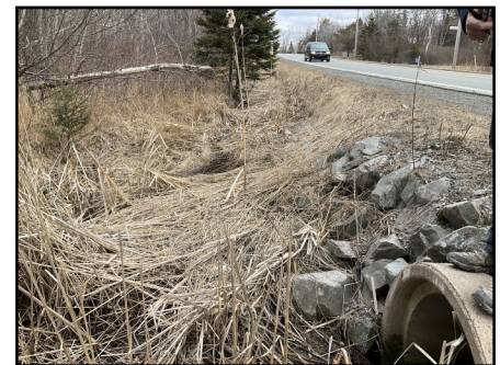
Photo 3: Overgrown vegetation in upstream channel
