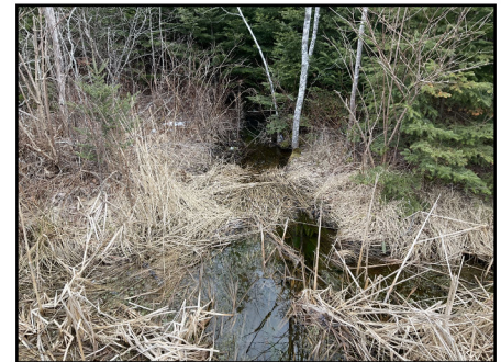
Photo 6: Downstream culvert with vegetation obstructions
