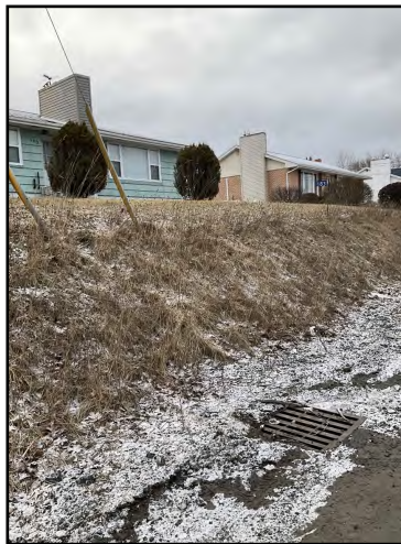
Photo 2: Catch basin on East side of shown under embankment at Civic Address 183.
