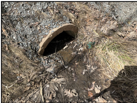
Photo 4: Outlet of culvert full half full of debris
