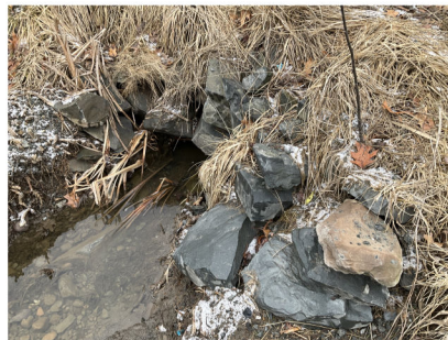
Photo 5: Outlet of culvert with approximately 180mm of water in outlet
