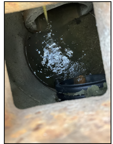
Photo 3: 600mm concrete pipe flowing NW from catch basin across the road from Home Hardware
