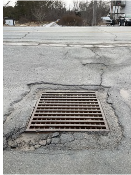
Photo 2: Catch basin connected to culvert in Post Office Parking Lot
