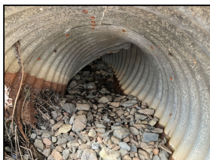
Photo 1: Inside of collapsed culvert
