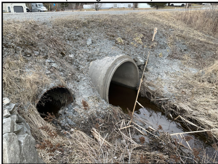
Photo 4: Outlet of culvert. Notice full flow from concrete culvert however steel culvert has debris buildup
