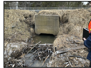
Photo 4: Outlet of culvert with debris buildup in channel
