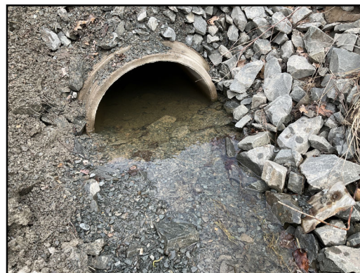
Photo 2: Gravel deposits at outlet of culvert
