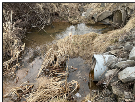
Photo 4: Vegetation growth at outlet of culverts
