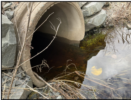
Photo 1: Outlet of pipe with approximately 100mm of standing water in pipe
