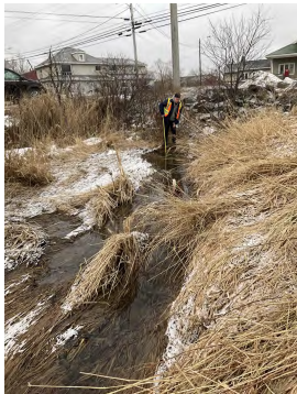
Photo 4: Downstream channel looking towards pipe
