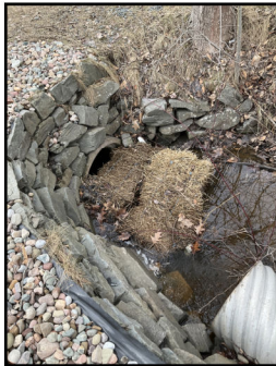
Photo 4: Bales blocking invert of culvert
