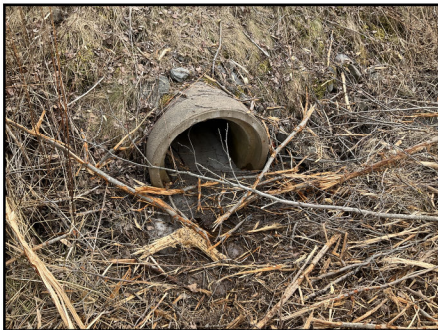
Photo 4: Debris in inlet from brush cutting operations
