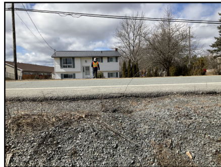
Photo 2: Shoulder of road above outlet
