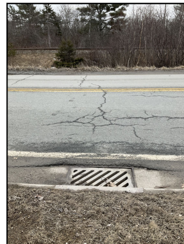
Photo 3: Catch basin connected to culvert with cracking across road
